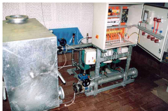
Fig. 4. Prototype pumping station implementing an energy-efficient control system
